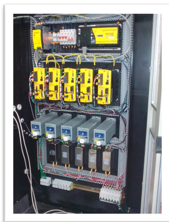
Figura 6. Panel de Control.
