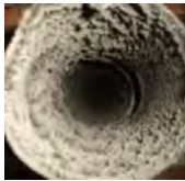
Fig. 2 Dust adhered in the duct
